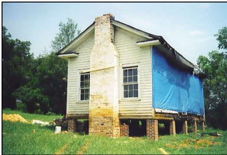
The house sitting on its new brick mounts, before it had a back.
